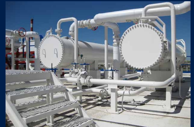
Heat Exchangers Pressure Vessels
